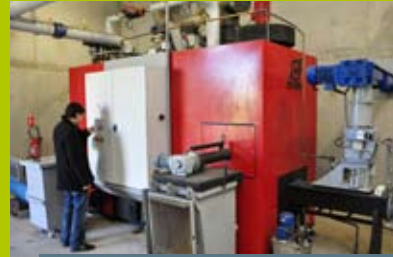
Automatic wood chip boiler
